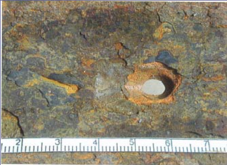
FIGURE 5 CLOSE-UP OF CORROSION PITTING AT PIPE BOTTOM
