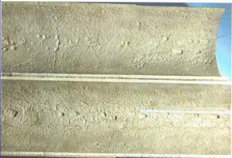
FIGURE 6 CORROSION PITTING ON SANDBLASTED INNER PIPE SURFACE
